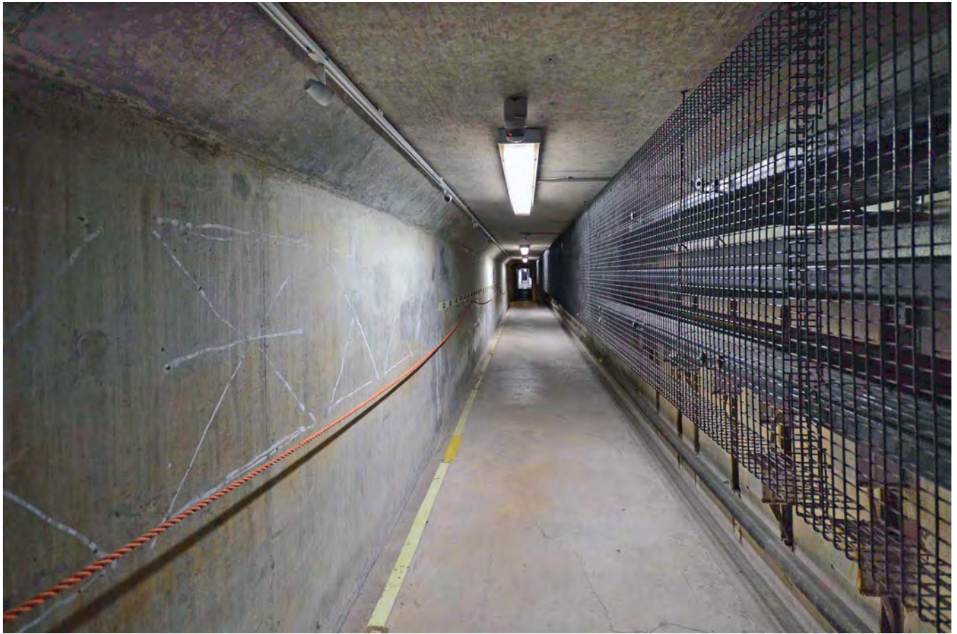
Under the middle of the river – downstream is the left. Service cables and hydraulics are neatly set behind weldmesh screen on the right
